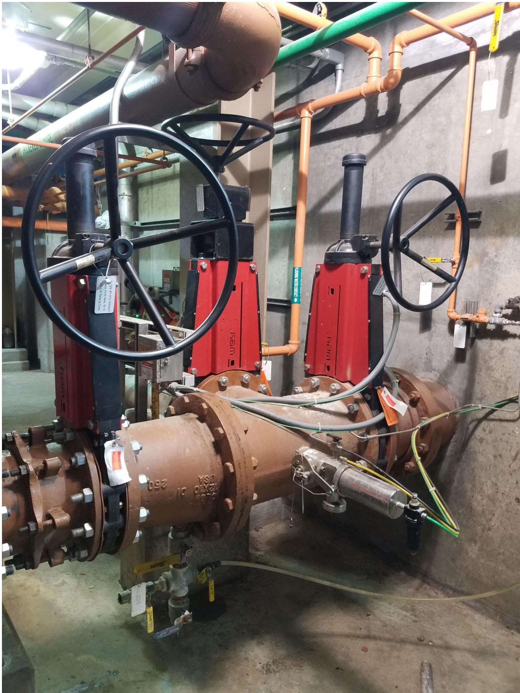
Wey VM bevel gear operated in a wastewater treatment plant in Ohio, USA.
